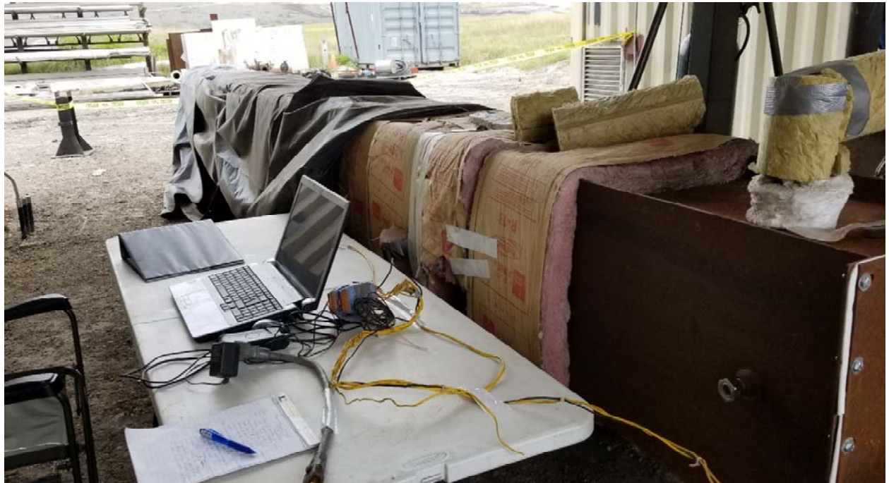
Photo 14: ITD/TO Control Panel
