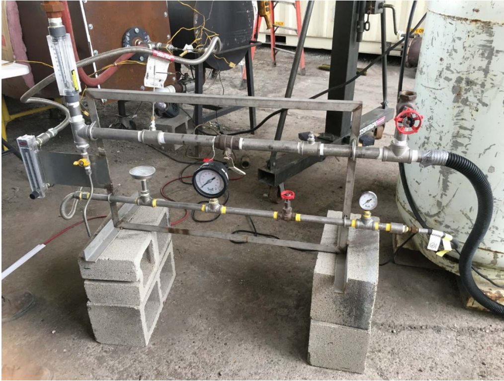
Photo 6: Air and Fuel Delivery Manifold
