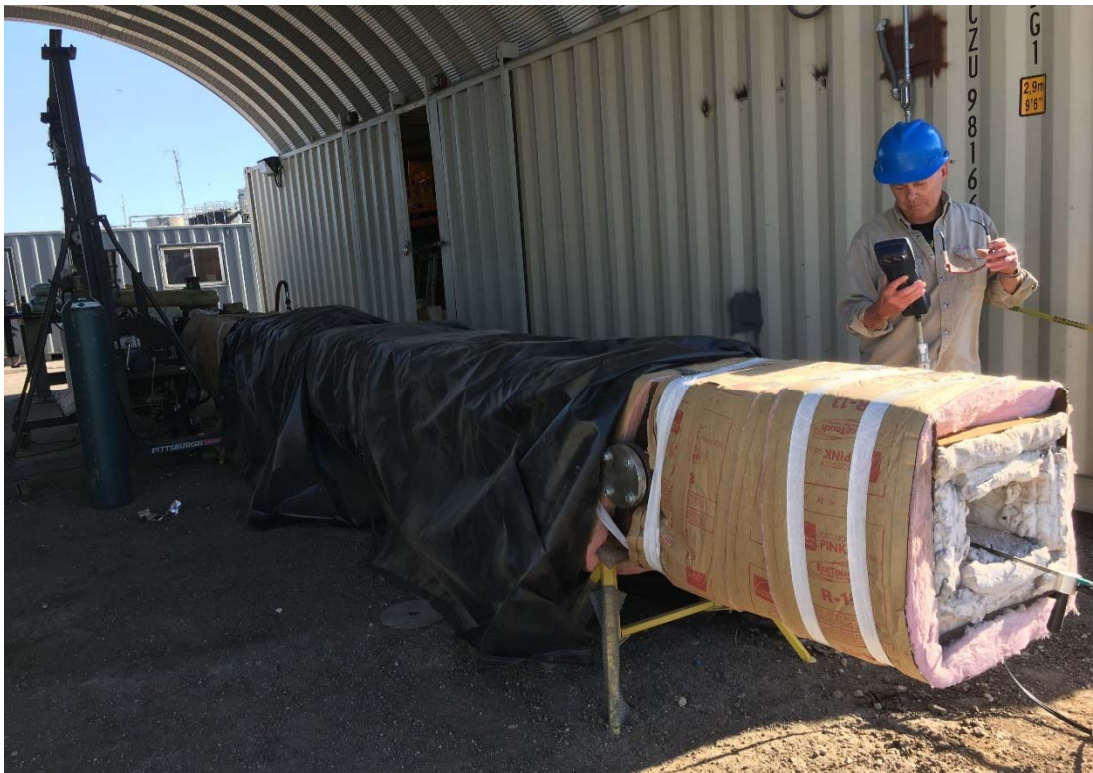
Photo 5: Checking Combustion Properties Inside Thermal Oxidizer
