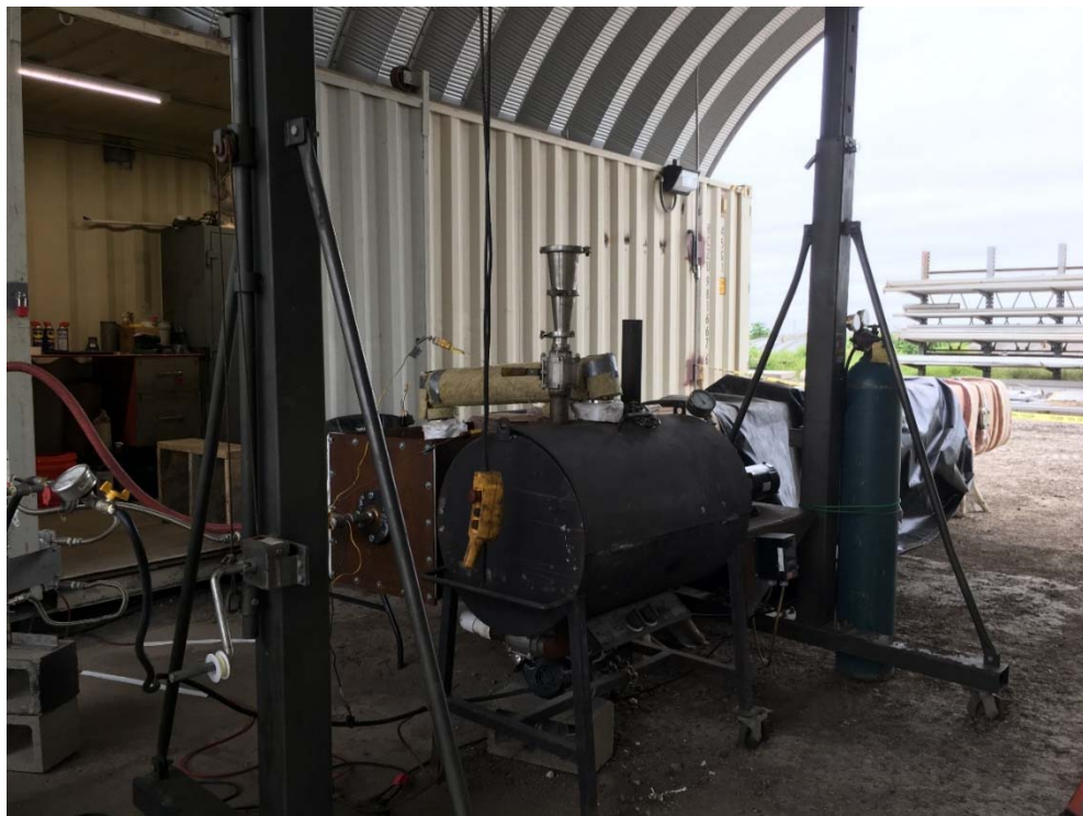
Photo 2: Indirect Thermal Desorption Unit and Thermal Oxidizer
