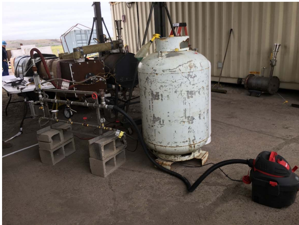
Photo 7: Additional View of Air and Fuel Delivery Manifold
